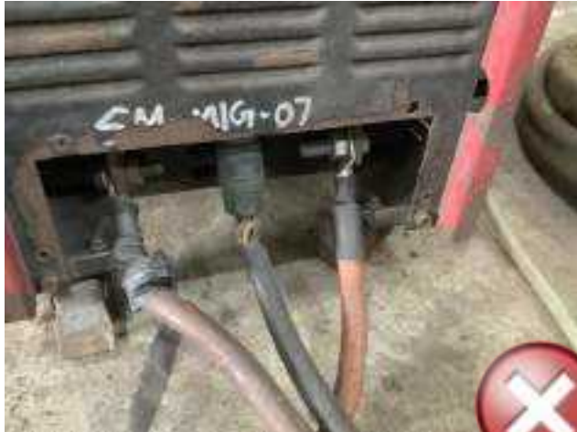
Electric welder with exposed connectors (conductors)
