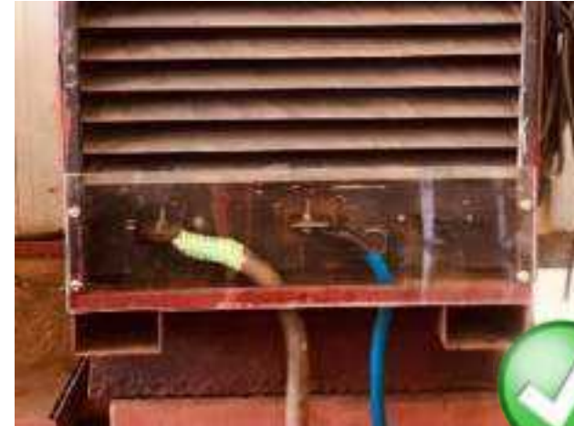
Connectors covered with insulating shield
